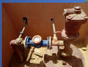
Water meter in Ponte Nova Borehole
