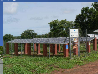
Bairro 4 Borehole Solar Panels
